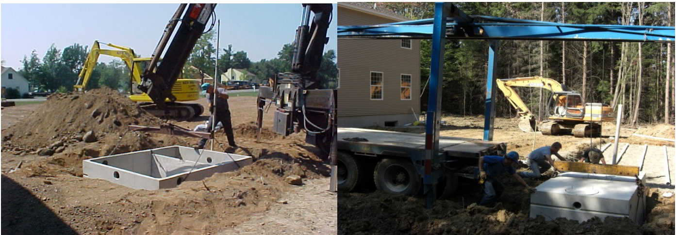
Above are examples of two tanks quickly and easily installed using native materials.
