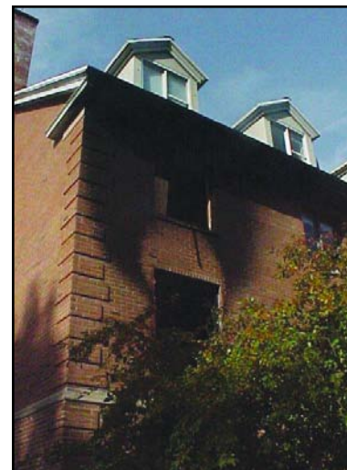
Burned out windows
