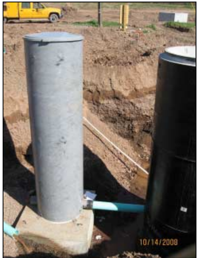
Metering manhole and pump station
