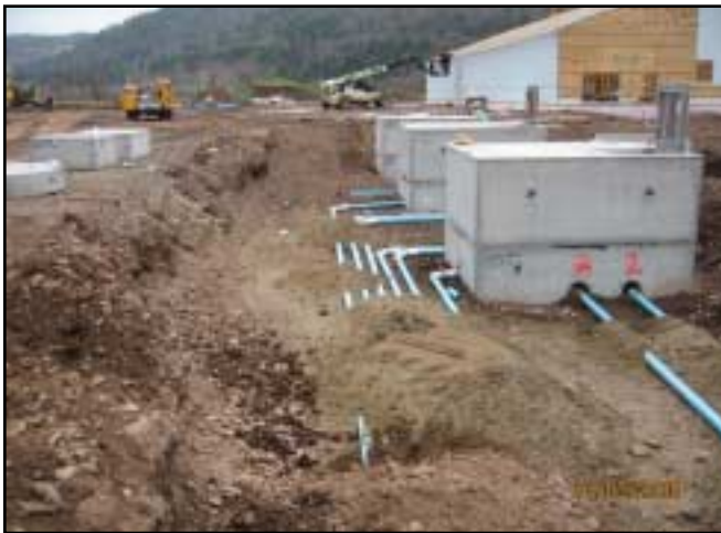
Absorption bed, valve vaults, and pump station
