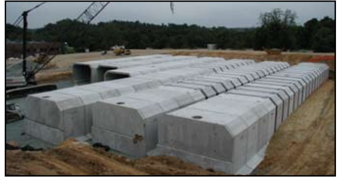
The SWM system consists of 6 barrels side by side, by 120' long each. Photos by: Rotondo Environmental Solutions LLC
