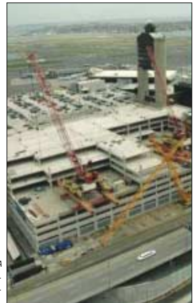
Logan International Airport Central Parking Garage Expansion, Boston, MA Architect: TAMS/Fennick/McCredie Architecture Ltd. Photo: Blakeslee Prestress Inc.
