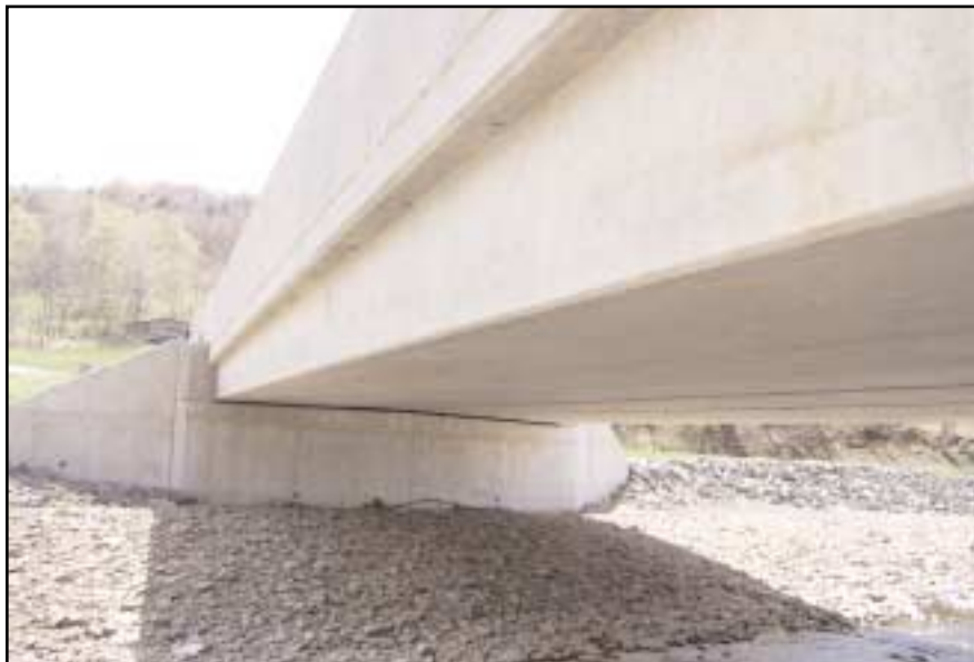
PA Wyoming Co., SR 3003, (GC: Glenn O. Hawbaker) 5 Spread Box Beams, 48" wide by 30" deep by 73.08' long (31.3 tons each)
