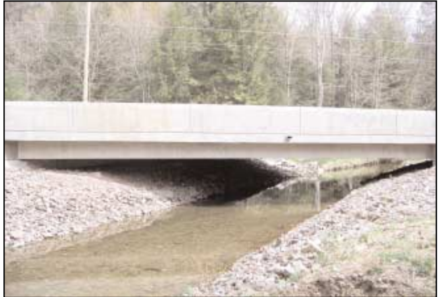
PA Luzerne Co., SR 118 (GC: Susquehanna Supply) Six 48” wide by 27” deep by 60’ long Spread Box Beams (24 tons each)
