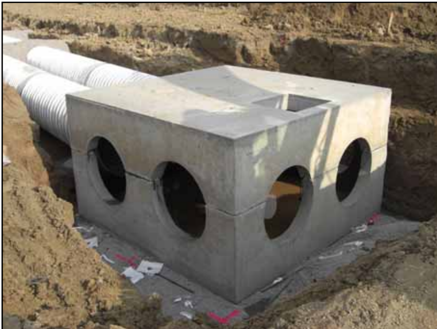
12' x 12' Junction Vault
