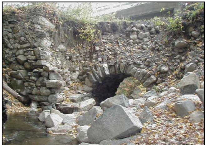
Partially Collapsed Stone Arch
