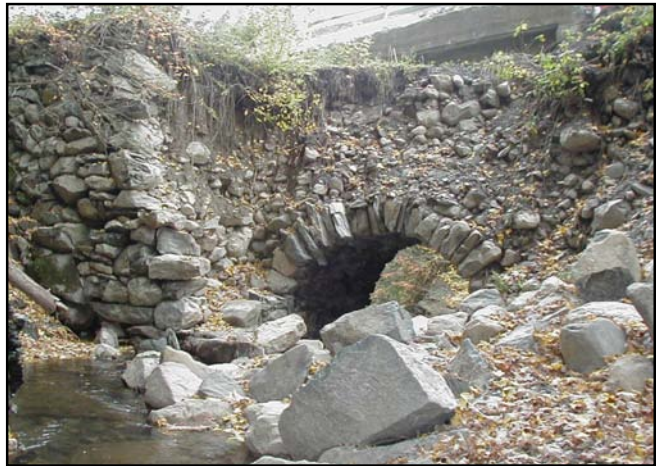
Partially Collapsed Stone Arch
