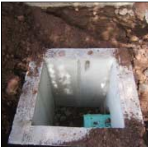
Catch basin installation in Village of Delhi, part of a storm water retrofit project
