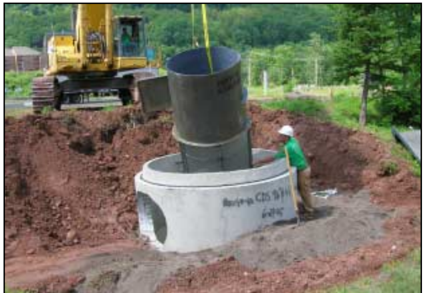
Installation of hydrodynamic separator, storm water control project, Hunter Town Highway Garage
