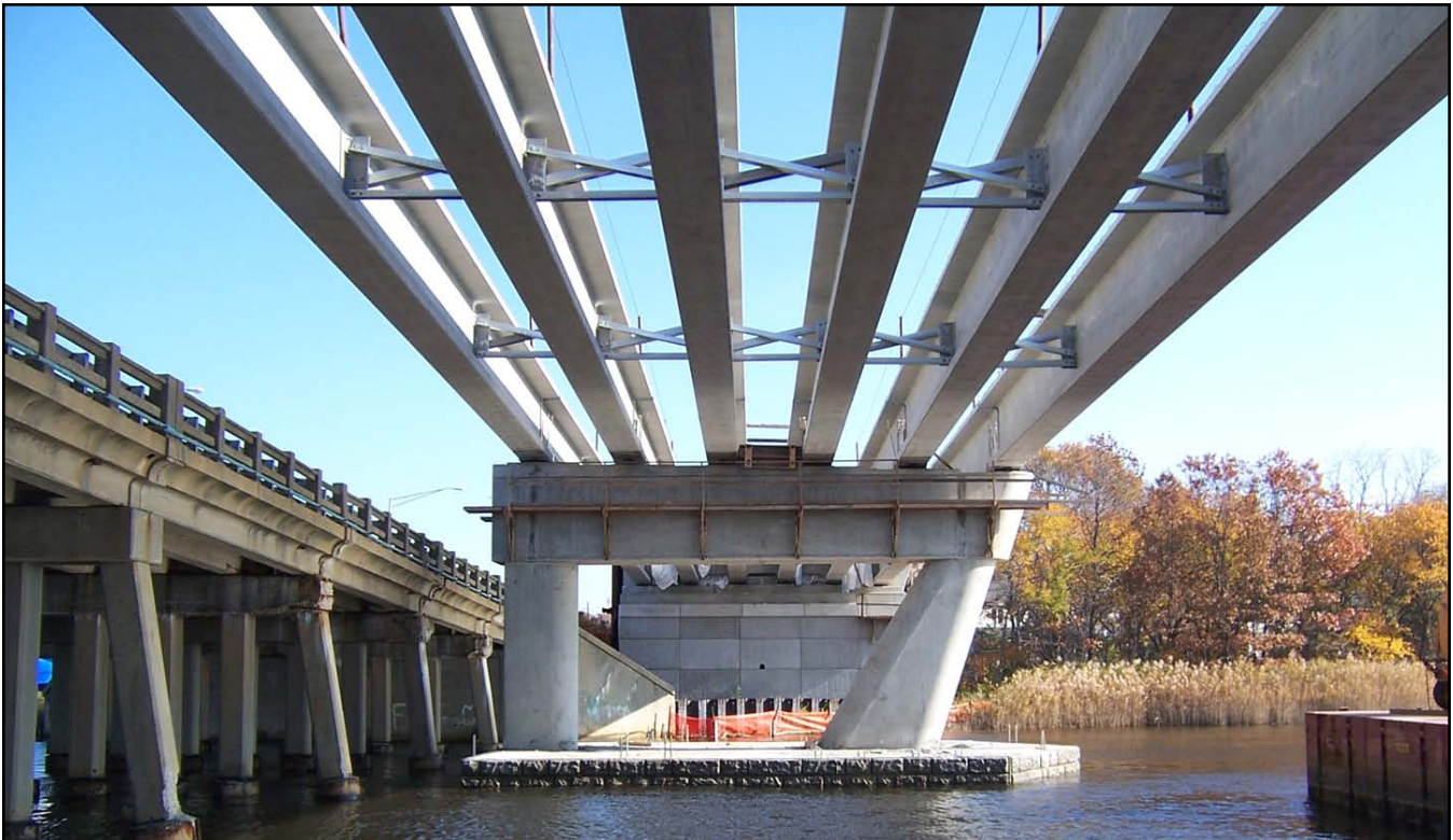
PCEF Bulb Tee Beams, Pier Caps and Columns installed over the Manasquan River
