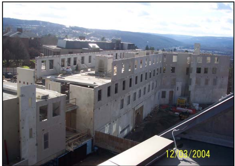
Bearing walls, clear span floors, and stair/elevator towers being installed Photo by Welliver McGuire
