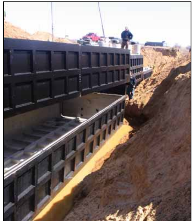
Equalization tank in foreground and five 10,000 gallon treatment tanks each with 9.0 FAST unit
