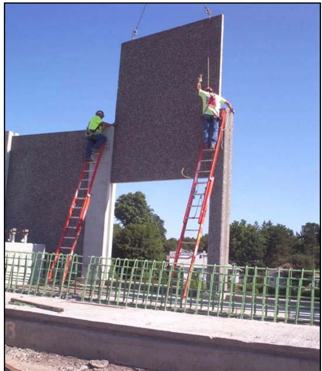
Simple, Fast Sound Wall Installation, I-86, Horseheads, NY Photo by: BVR Construction Co, Inc.
