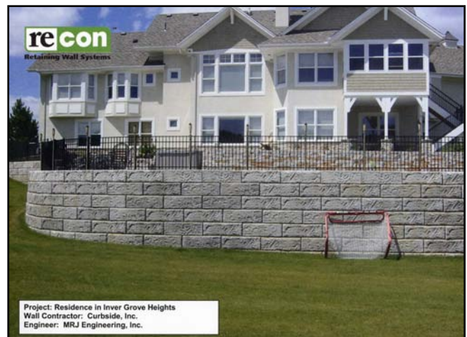
Project: Residence in Inver Grove Heights Wall Contractor: Curbside, Inc. Engineer: MRJ Engineering, Inc.
