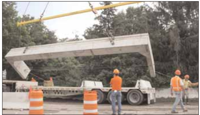
Lift and Roll of 39' 6" three-sided bridge unit Photo by Kistner Concrete Products
