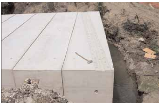
Keyway with rebar couplers cast on a skew to accommodate highway layout
