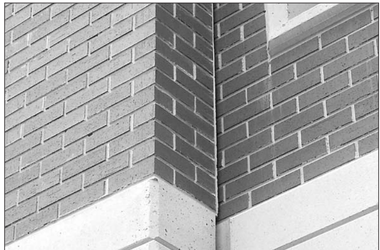
Hoboken garage showing base of column, spandrel beam inset, and bottom of window. Photo by Unistress.
