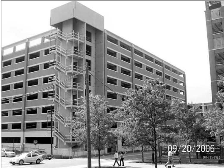
Erection of precast elements on Hoboken Cove garage in Hoboken, NJ was completed in September. Spandrels and columns feature thin set brick, highlighted by buff colored details to match adjacent condominiums. Photo by Unistress.
