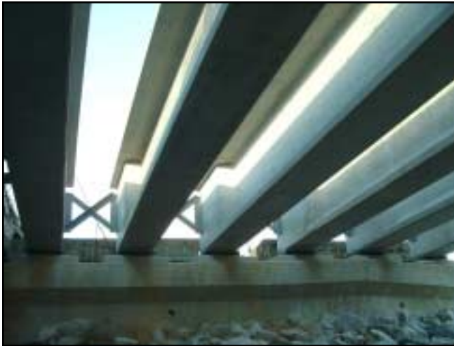
Route 17/Wallkill River Project Outer Segments With Enlarged Web End Blocks, Shown in Place on Old Abutments
