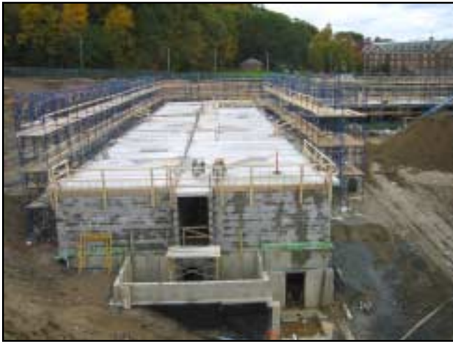
Construction underway for new student apartment complexes Photos by J. P. Carrara & Sons
