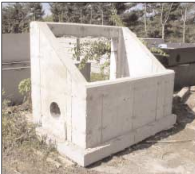
Outlet Control Structure for Detention Pond Photo by Eastern Precast
