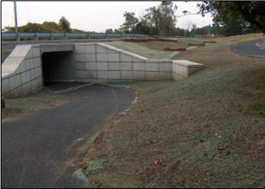
Storm water is collected on the upstream end, and piped to the downstream side of the underpass.
