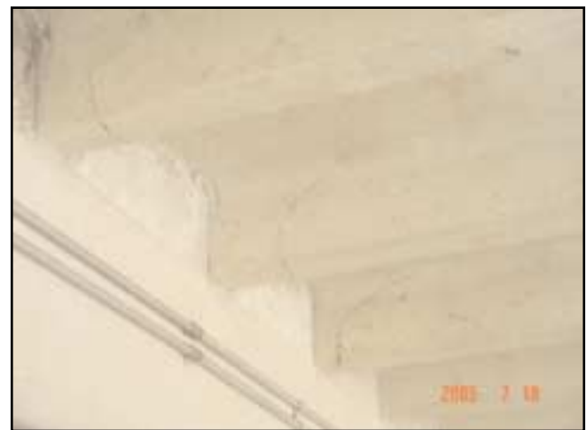
Locust Street – Cracks in ends of double tees (photos by W.S.A.)
