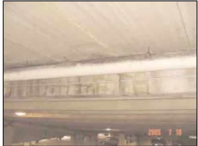
Chestnut Street – Cracks in precast concrete beam
