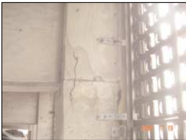
5th Street – Cracked beam-column connection
