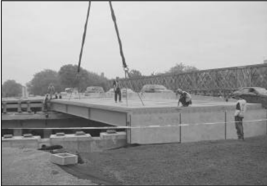
Main span bridge units included semi-integral abutments with overhung end closure walls, eliminating expansion joints from the bridge All photos by Fort Miller
