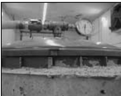
Gage indicating vacuum pulled
