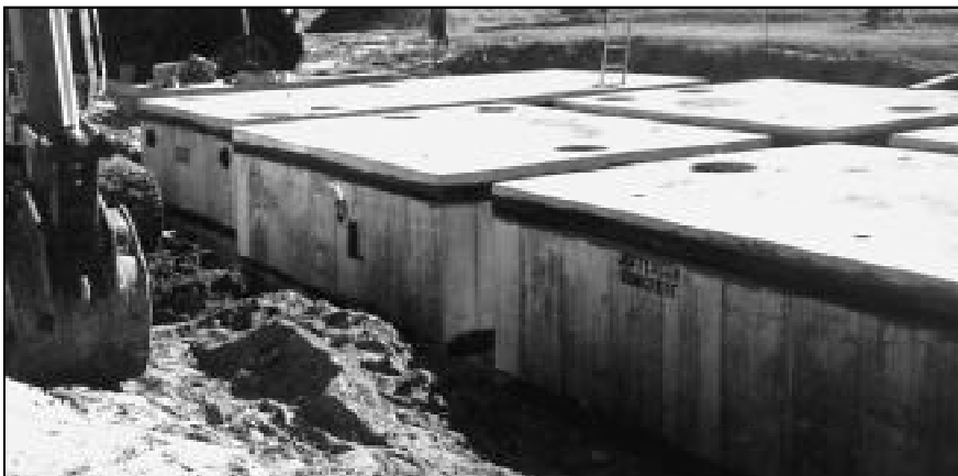
Top photo shows installation of mastic seal between wall and top slab on equalizer tank. Bottom photo shows tanks with joint wrap in place ready for back fill. photos by Jefferson Concrete
