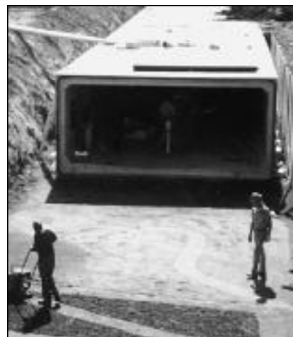
Precast box members are installed for an underground storm water storage tank.
