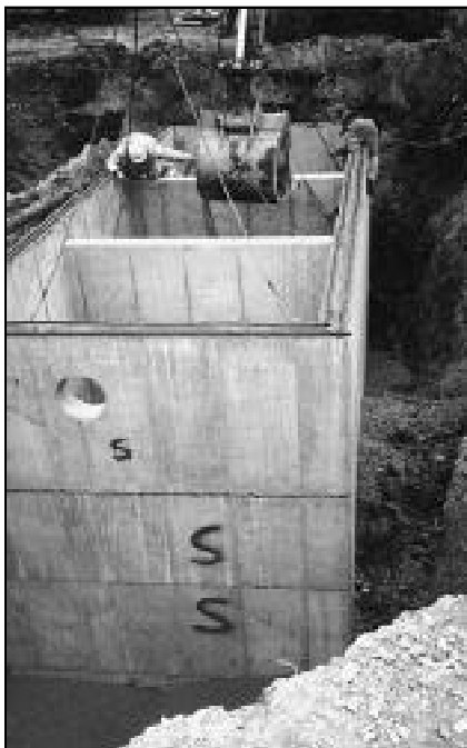
Workman install top riser segment on new precast water tank. photo by Jefferson Concrete
